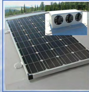
170 Watt Roof Mounted Solar Panel
